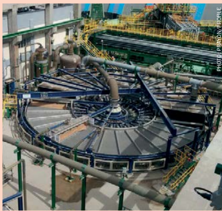
Above: Profile's model 30-220 tilting pan filter with a total surface area of 220 m 2 . Installed at OCP's Jorf Lasfar phosphates production complex in Morocco.
