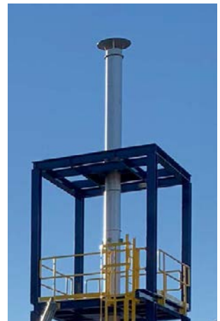
The addition of an H 2 S scrubbing system ensures that stack emissions comply with the most stringent regulations globally.
