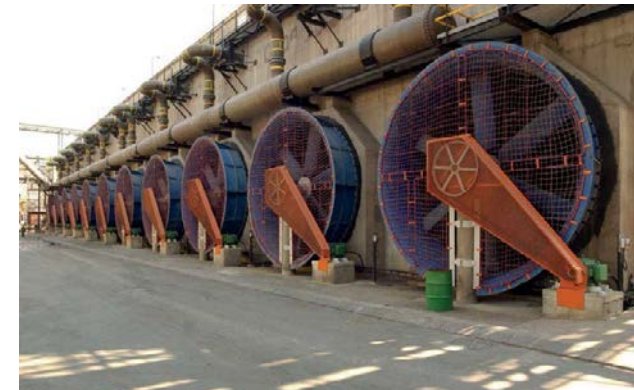
A line of eleven cooling tower cells at a phosphoric acid plant, each cell having its own belt-driven, six-blade fan.
