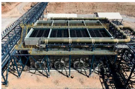
Fig. 6: Forced draft cooling towers cells in a back-to-back layout.
