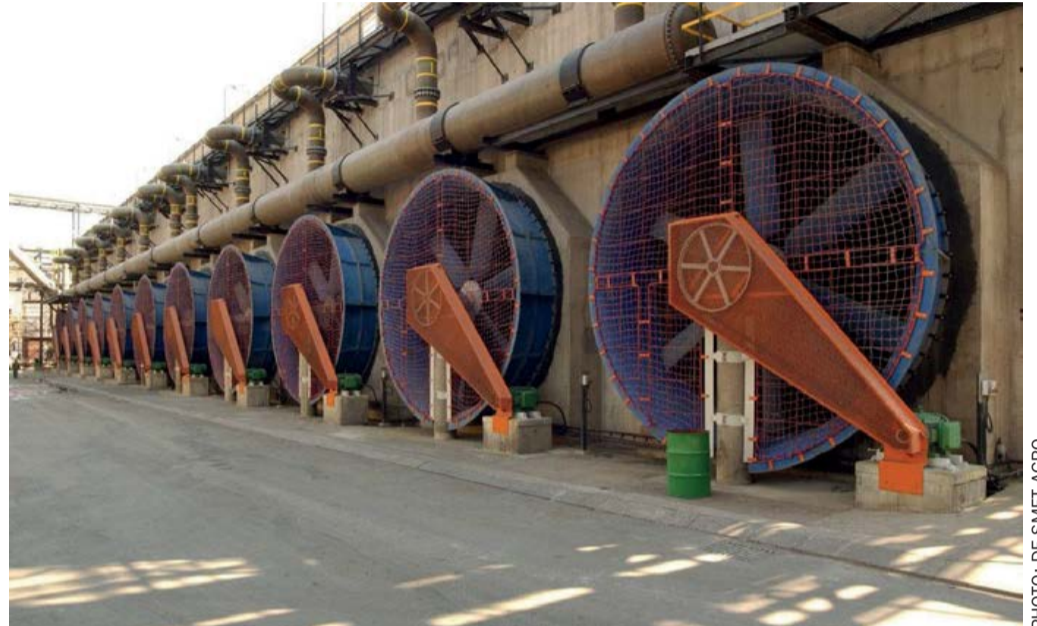
A line of eleven cooling tower cells at a phosphoric acid plant, each cell having its own belt-driven, six-blade fan.
