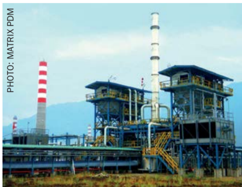
Above: Two Devco II wet prilling units, central China. These 8,600 t/d capacity units have a space-efficient, modular design.
