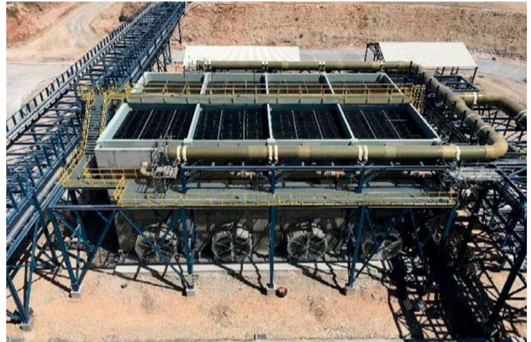
Fig. 6: Forced draft cooling towers cells in a back-to-back layout.
