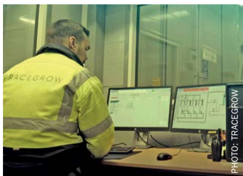
Control room of Tracegrow’s battery recycling and fertilizer manufacturing plant in Finland.
