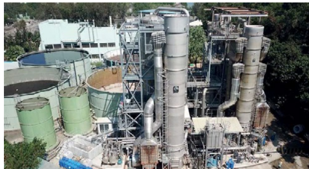
The 3,250 m 3 /day rated thermal ammonia stripping plant at the West New Territories (WENT) landfill site, Hong Kong, China.
