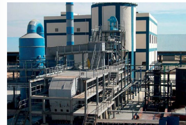
Fig. 4: Complete Broadfield process unit, Aswan, Egypt.
