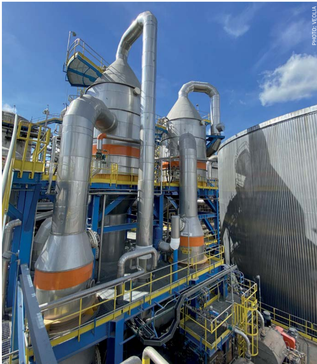
Veolia's HPD® ECRP™ (Enhanced Chloride Removal Process) system.
