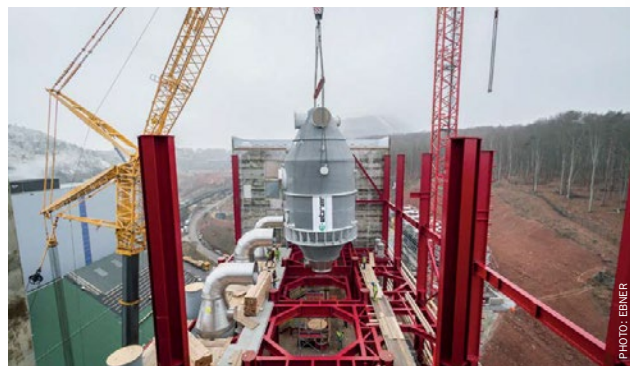
Ebner designed, manufactured and erected this evaporation and crystallisation plant for K+S.
