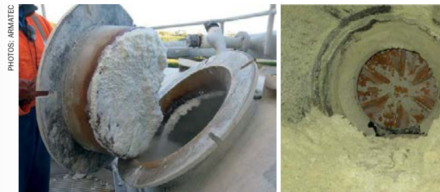
Silica deposits (left) are a natural and unavoidable by-product of scrubbing. These need to be carefully managed to avoid blocking pipes, ducts and fans (right).
