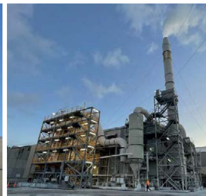
Case study 2: Phase 1 of the SSP scrubber upgrade (left) helped the client win an environmental award. The recently completed phase 2 of the upgrade (right) has future-proofed the site for increased production.
