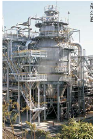
Reactive crystalliser unit used in ammonium sulphate production.
