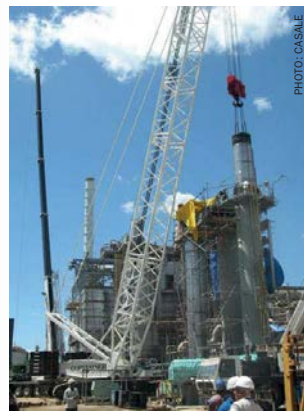
Casale's revamp of the CF Braun ammonia plant focused on the reduction of carbon dioxide emissions.
