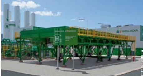
Puertollano green hydrogen plant, Spain. PHOTO: IBERDROLA
