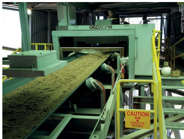
North American Geoscan-M installation for monitoring beneficiated phosphate – with a TBM moisture analyser in the foreground.
