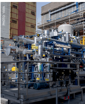
The 24MW renewable hydrogen plant at Herøya Industrial Park in Porsgrunn, Norway, is the largest of its kind currently operating in Europe.
