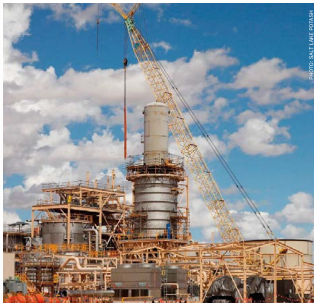
Erection and installation of the SOP crystallisation plant at Lake Way, Western Australia.
