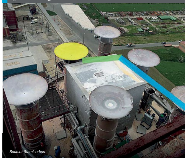
Fig. 6: Pilot testing Jet Venturi scrubber
