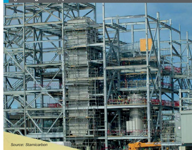
Fig. 3: The granulator, quench and MMV scrubber installed at DGC
