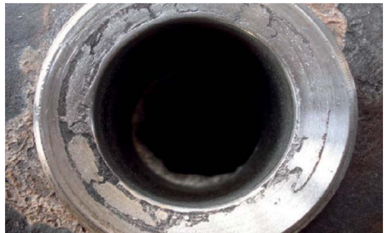
Fig. 4: Signs of crevice corrosion of a stainless steel flange face.
