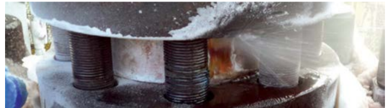
Fig. 5: A typical leak of a lens ring flange connection.
