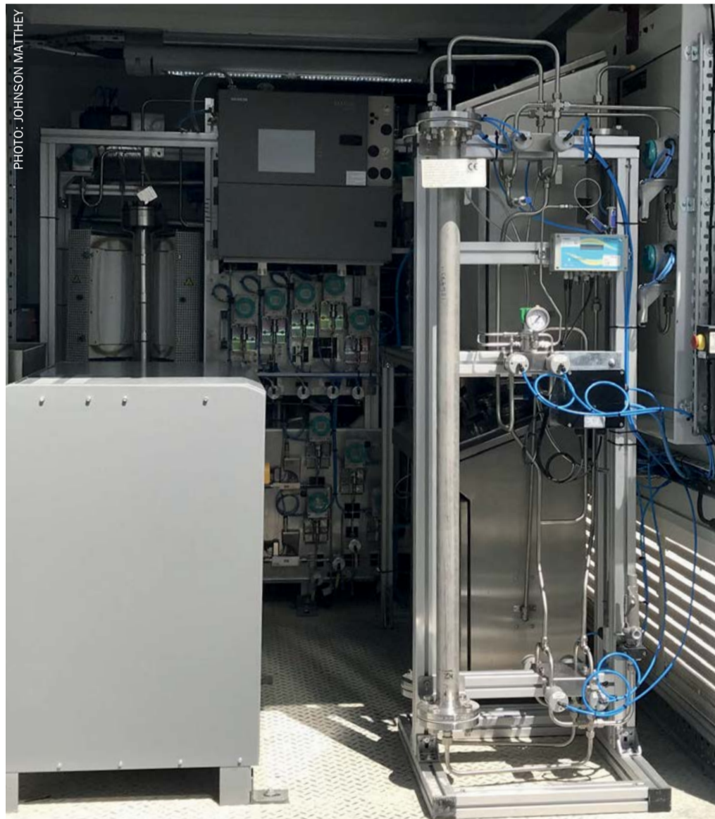
Fig. 4: Green ammonia demonstrator plant in which KATALCO 74-1 was installed.
