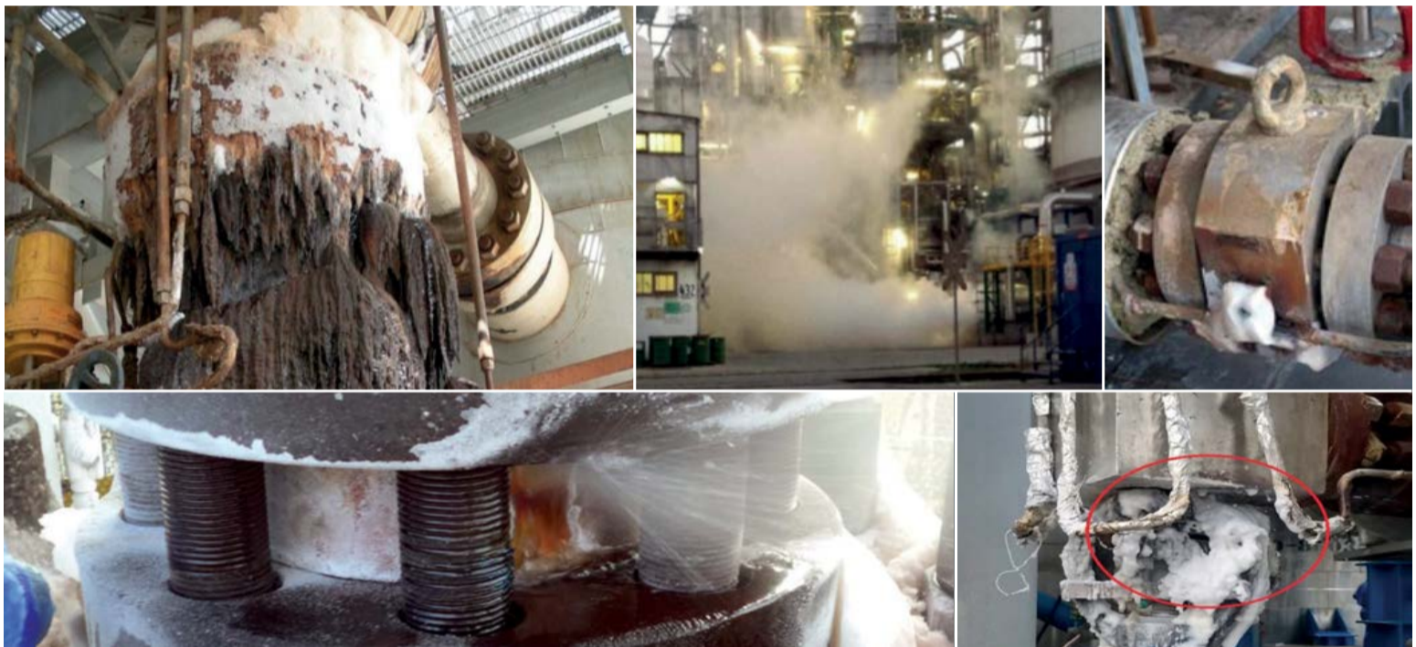
Several examples of leaks in urea plants.
