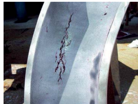
Fig. 4: Cracks in a high-pressure carbamate gas line.
