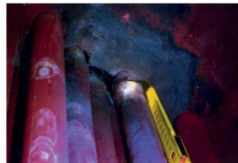
Fig. 2: Severe corrosion of the carbon steel tubesheet due to a leak in a tube.
