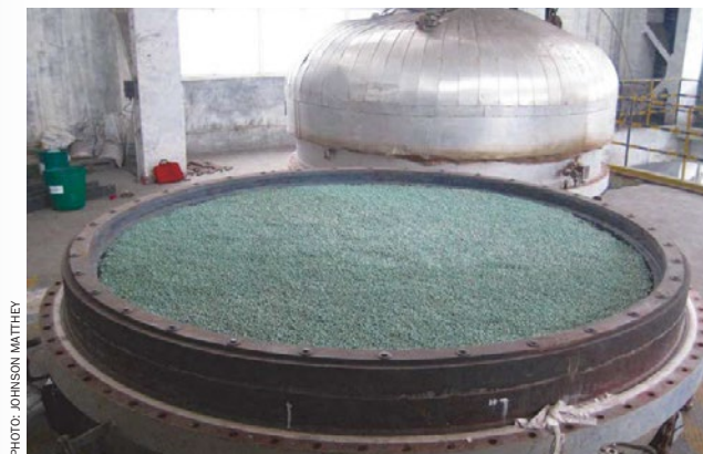
Fig. 3: Secondary catalyst bed of Yara 58-Y1 immediately below gauze burner hood.
