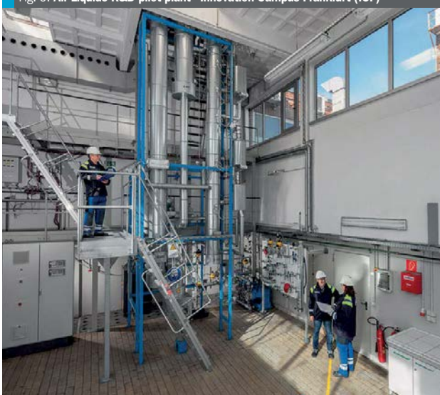
Fig. 9: Air Liquide R&D pilot plant - Innovation Campus Frankfurt (ICF)
