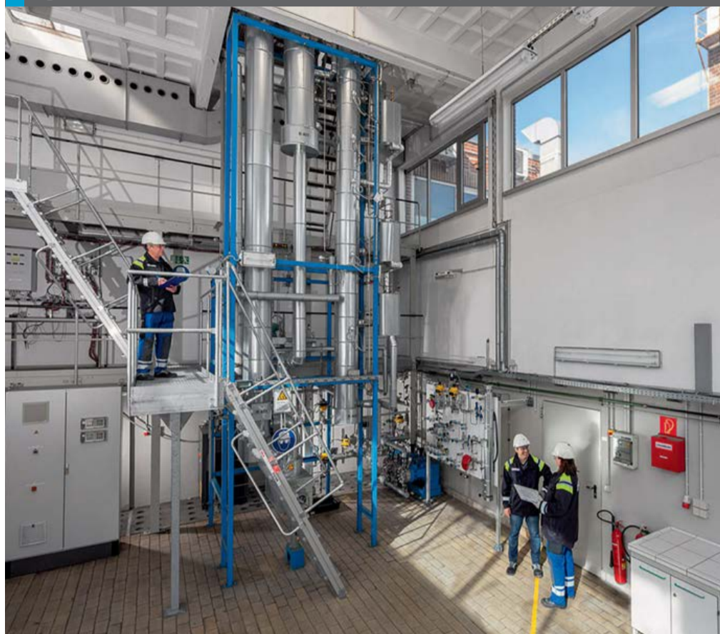
Fig. 9: Air Liquide R&D pilot plant - Innovation Campus Frankfurt (ICF)
