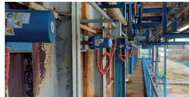
Fig. 10: Photo of installed ZoloSCAN sensor heads on the reformer at Yara Le Havre.
