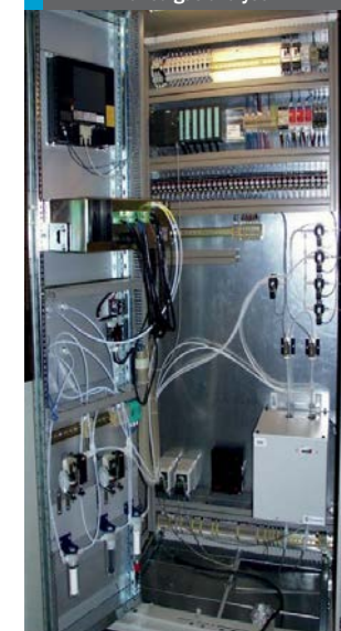
Fig. 1: Conventional cold extractive infra-red gas analyser
