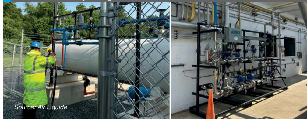
Fig. 4: Ammonia tank at ICD being filled by Airgas personnel (left). Flow control skids for NH 3 and H 2 (right).
