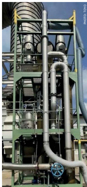
Fig. 3: Side view of pilot plant
