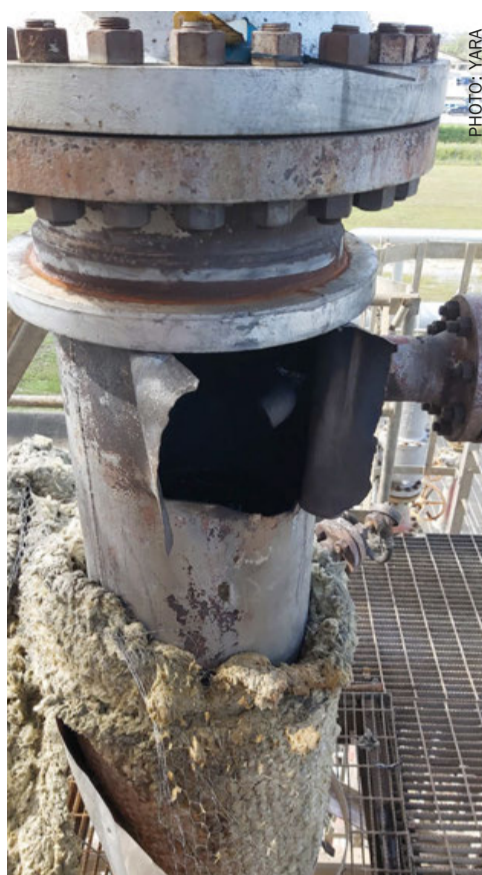
Fig. 4: Close view of the failed stripper
