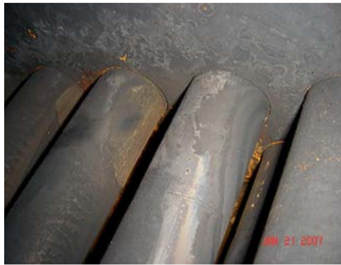
Fig. 12: Corrosion at 6 o'clock on condenser inlet tubesheet.
