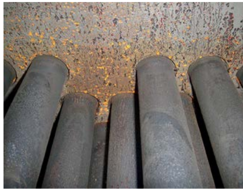
Fig. 13: Oxygen pitting on condenser inlet tubesheet.
