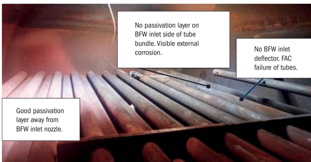
Fig. 2: Flow-accelerated corrosion caused by disturbance at the BFW Inlet
