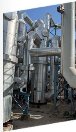
Sulphuric Acid Plant, Commissioned Oct 2020
