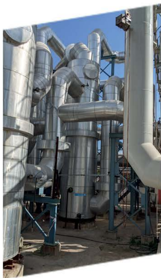
Sulphuric Acid Plant, Commissioned Oct 2020
