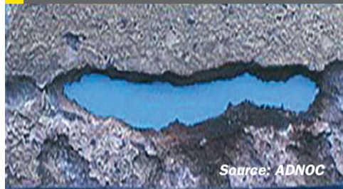
Fig. 5: Internal deep corrosion
