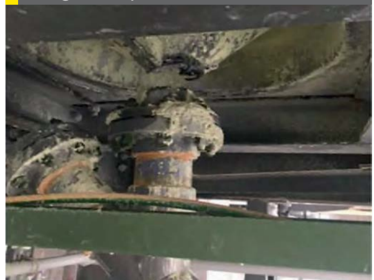
Fig. 2: Bottom of stack completely corroded at sulphur granulation plant
