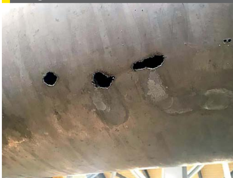
Fig. 1: Corroded scrubber outlet duct at sulphur granulation Plant
