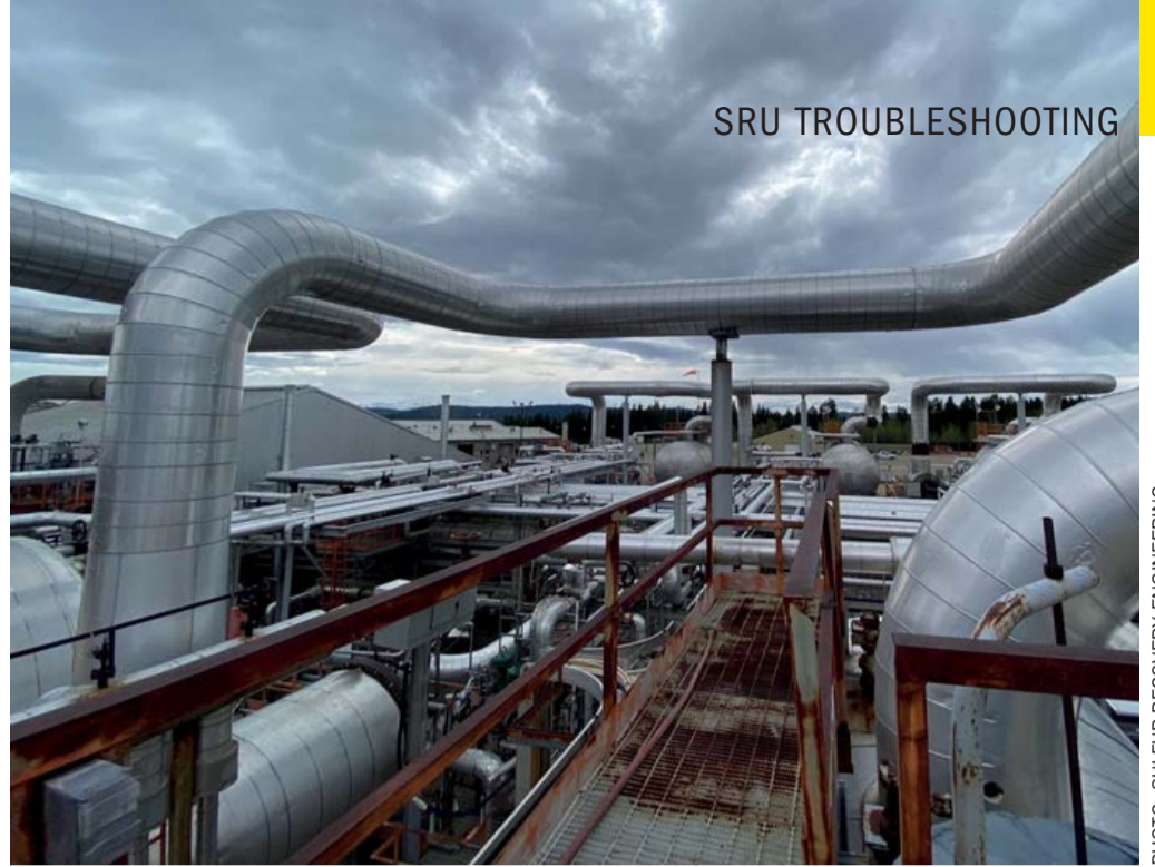
Direct fired reheater outlet line to the downstream converter.
