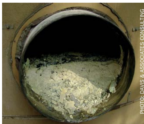
Fig. 2: Sulphate and scale can plug the drain line.
