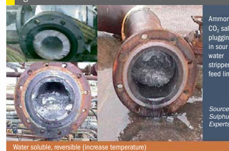
Fig. 3: Ammonia salts in SRU feed lines
