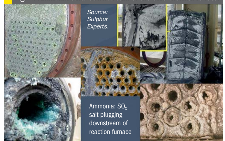
Fig. 4: Ammonia salts downstream of the SRU thermal reactor
