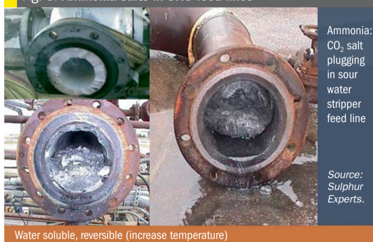
Fig. 3: Ammonia salts in SRU feed lines
