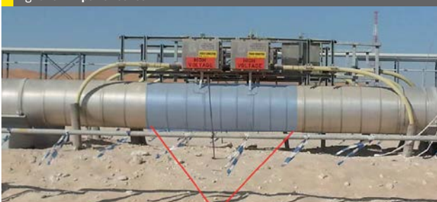
Fig. 5: SEET power boxes
