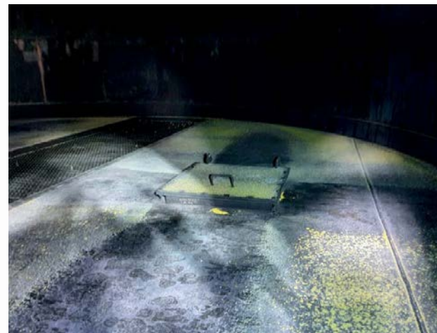
Fig. 5: Inspection showing the hatch with only 2 out of 16 bolts, and clear pattern of gas having passed through.
