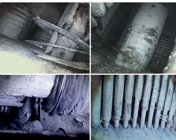
Fig. 3: Corrosion on the finned tube of the 1st economiser.
