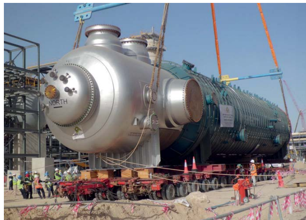
Fig. 2: 2nd generation incinerator burner installed at Habshan 5
