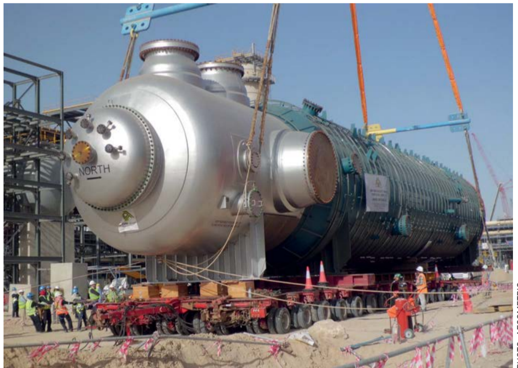
Fig. 2: 2nd generation incinerator burner installed at Habshan 5
