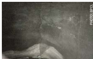
Fig. 8: Loose mesh on refractory wall
