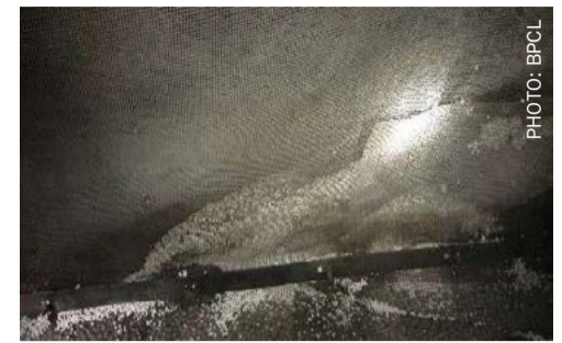
Fig. 7: Loose mesh near bottom grid
