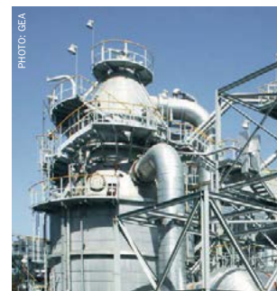
Operational GEA crystalliser at a fertilizer production plant.
