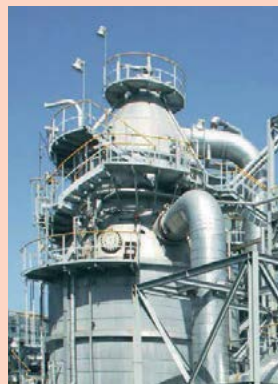
Operational GEA crystalliser at a fertilizer production plant.
