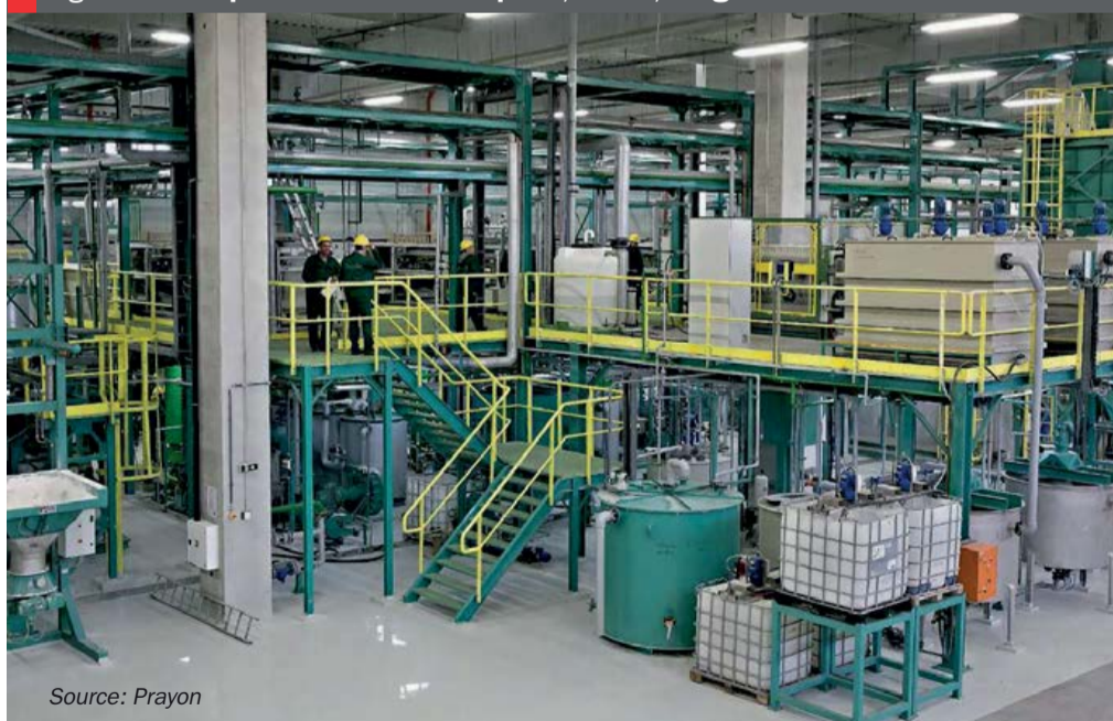
Fig. 6: Technophos semi-industrial plant, Varna, Bulgaria
