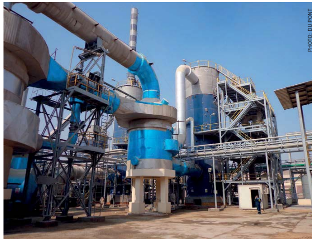
AZFC's Unit 6 after the revamp project.
