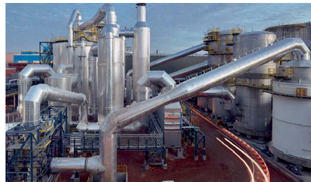
Mazidagi’s sulphuric acid plant.
