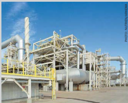
Nutrien's Aurora phosphate production complex in North Carolina. The site of an innovative new plant that will produce anhydrous hydrogen fluoride (AHF) from fluorosilicic acid (FSA).
