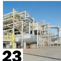
20 EMT urea hopper, ISAOSA blending plant, Mexico
