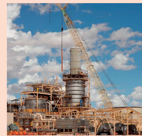
Erection and installation of a SOP crystallisation plant at Lake Way, Western Australia.
