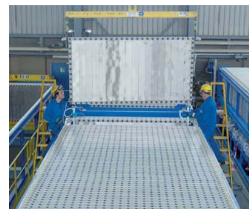
Electrolyser installation by Thyssenkrupp Steel.
