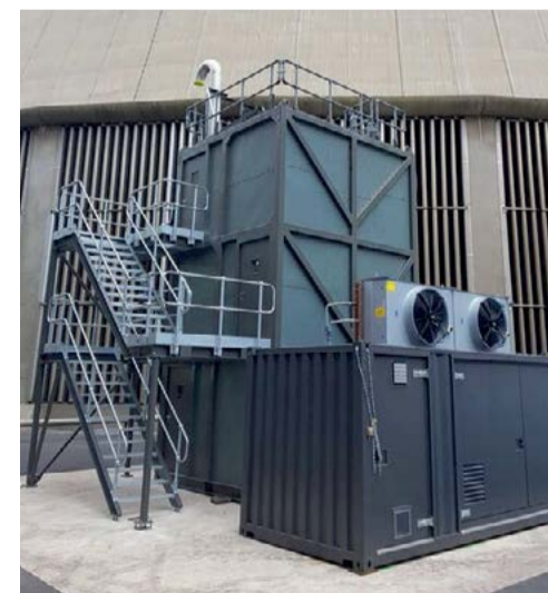
The MefCO 2 module on-site at Niederaussem, Germany.
