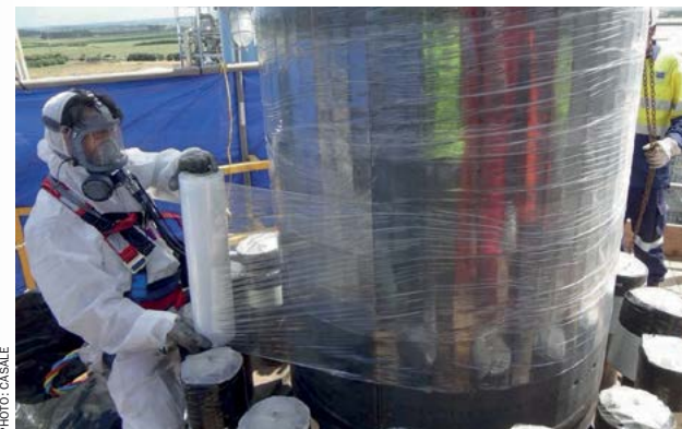
Fig. 5: Lifting of basket full of active catalyst purged with nitrogen – plastic wrapping to avoid the catalyst coming into contact with oxygen.
