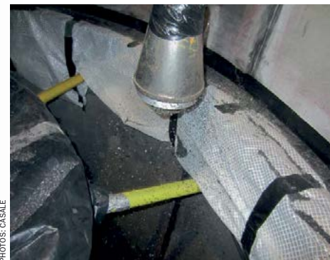
Fig. 3: Casale dense loading tool spreading the catalyst in the bed.
