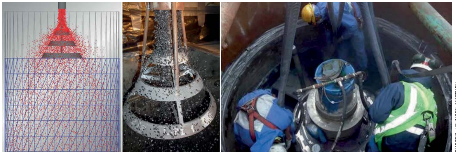
Fig. 5: Loading of tkIS uhde process ammonia converters.
