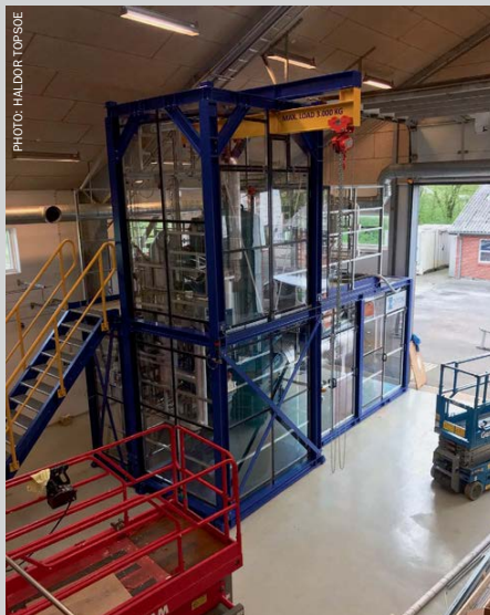
Topsoe's new biogas to methanol demonstrator plant.
