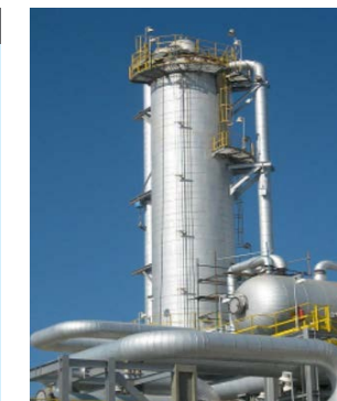
Fig. 7: MRF-Z® reactor for Oman Methanol Company.
