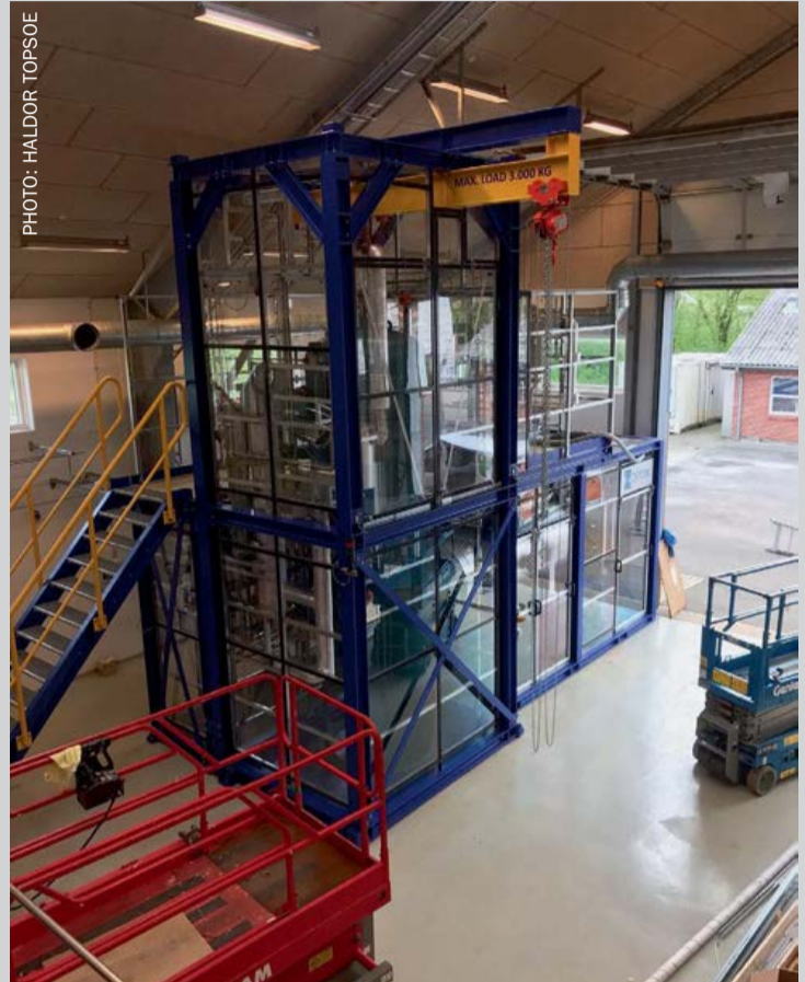
Topsoe's new biogas to methanol demonstrator plant.
