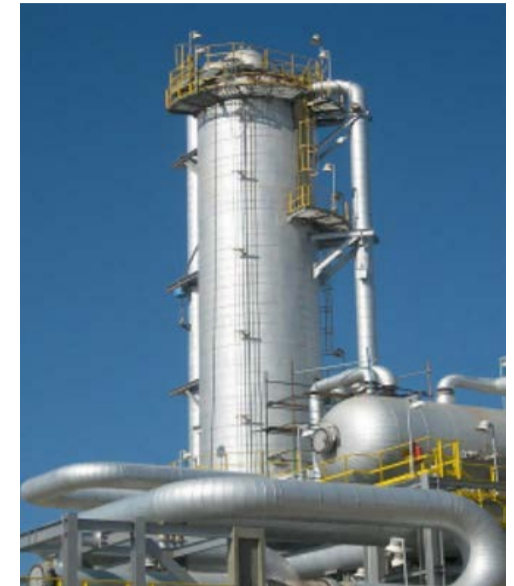
Fig. 7: MRF-Z ® reactor for Oman Methanol Company.
