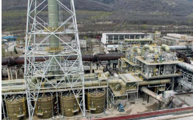
The gas cleaning section at the Pirdop smelter.
