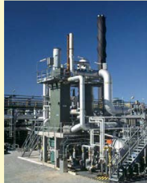
A WSA plant such as this treat tail gas from the Claus unit to achieve more than 99.9% sulphur removal efficiency (SRE).
