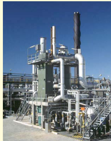
A WSA plant such as this treat tail gas from the Claus unit to achieve more than 99.9% sulphur removal efficiency (SRE).
