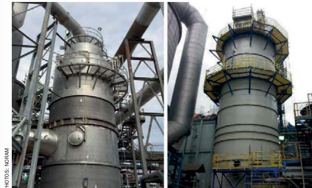
Fig. 6: NORAM acid towers. Project A (left). Project B (right).
