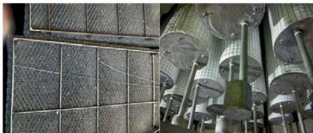
Fig. 3: Mist Eliminators. Project A (left): mesh pads. Project B (right): Brownian diffusion candles.
