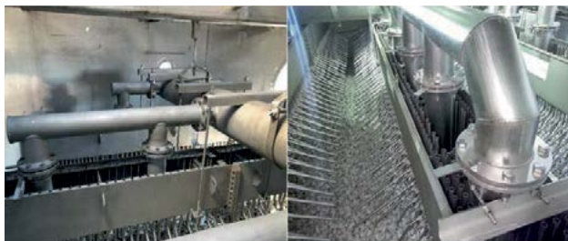
Fig. 4: Trough distributor. Project A (left): alloy tower. Project B (right): brick-lined tower.
